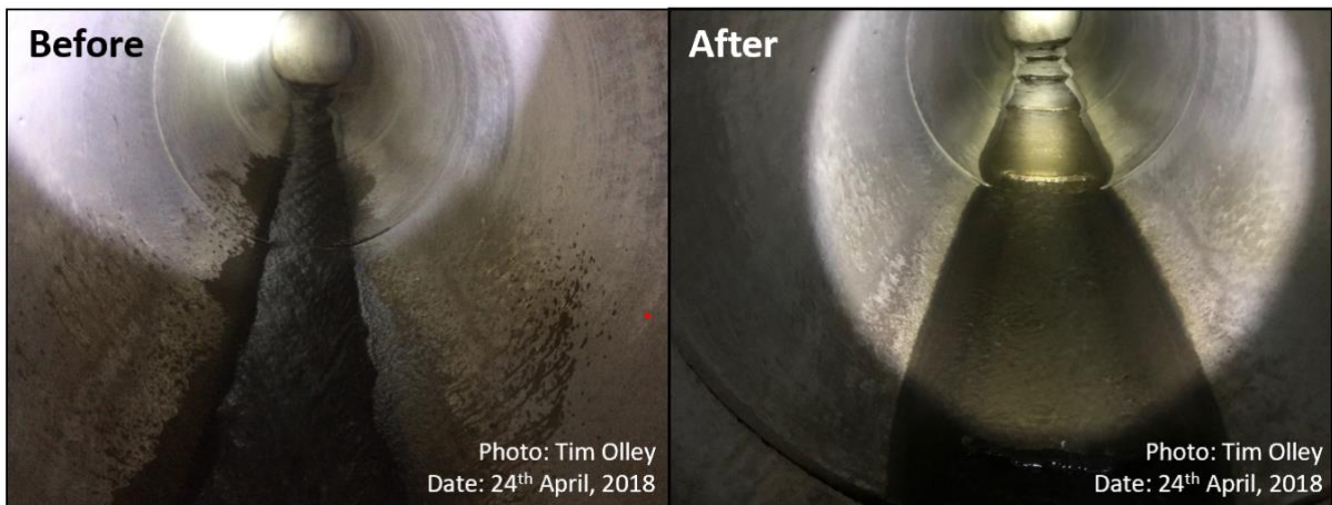
Figure 2. Lower section of the Reservoir Creek culvert before and after Flexi-baffle installation.
