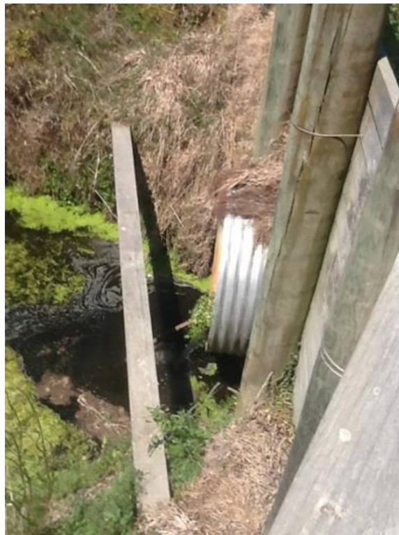
Figure 1: Outlet prior to remediation
